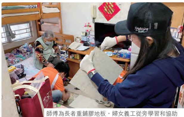
師傅為長者重鋪膠地板，婦女義工從旁學習和協助 Resurfacing rubber flooring for the elderly
